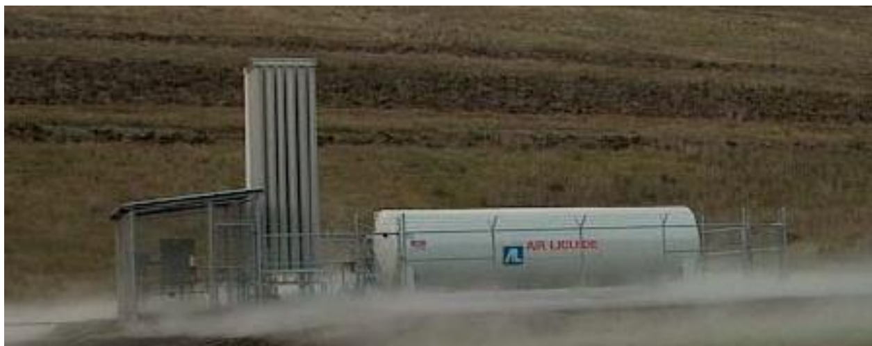
Figure 40. Oxygen tank and vaporizer for a diffused oxygen system
