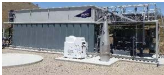
Figure 3-1 Single Train MBR Treatment Module
