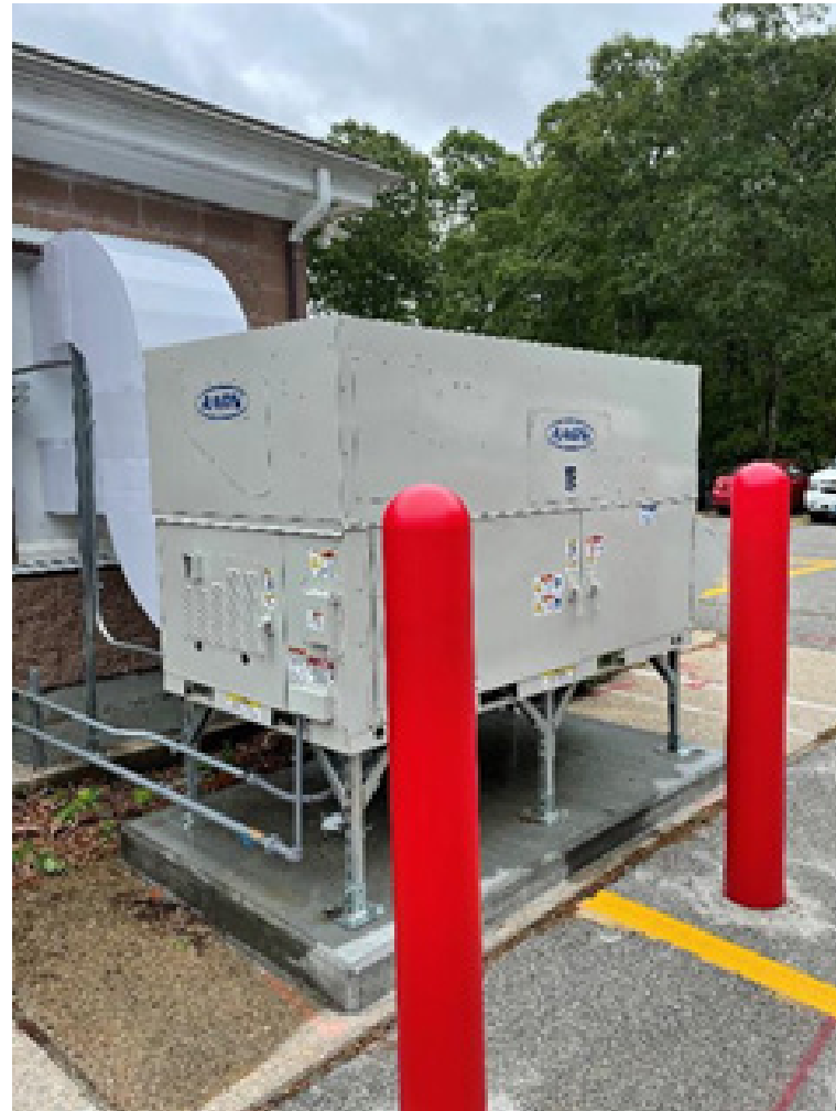
Outdoor Energy Recovery Ventilator (ERV)
