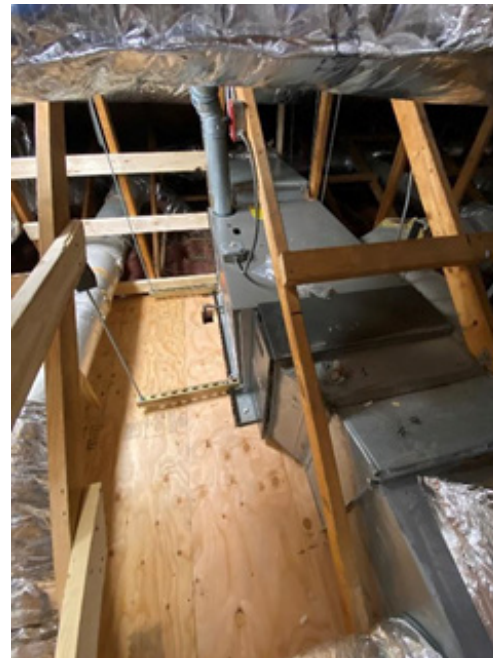
Furnace Unit in Attic Space
