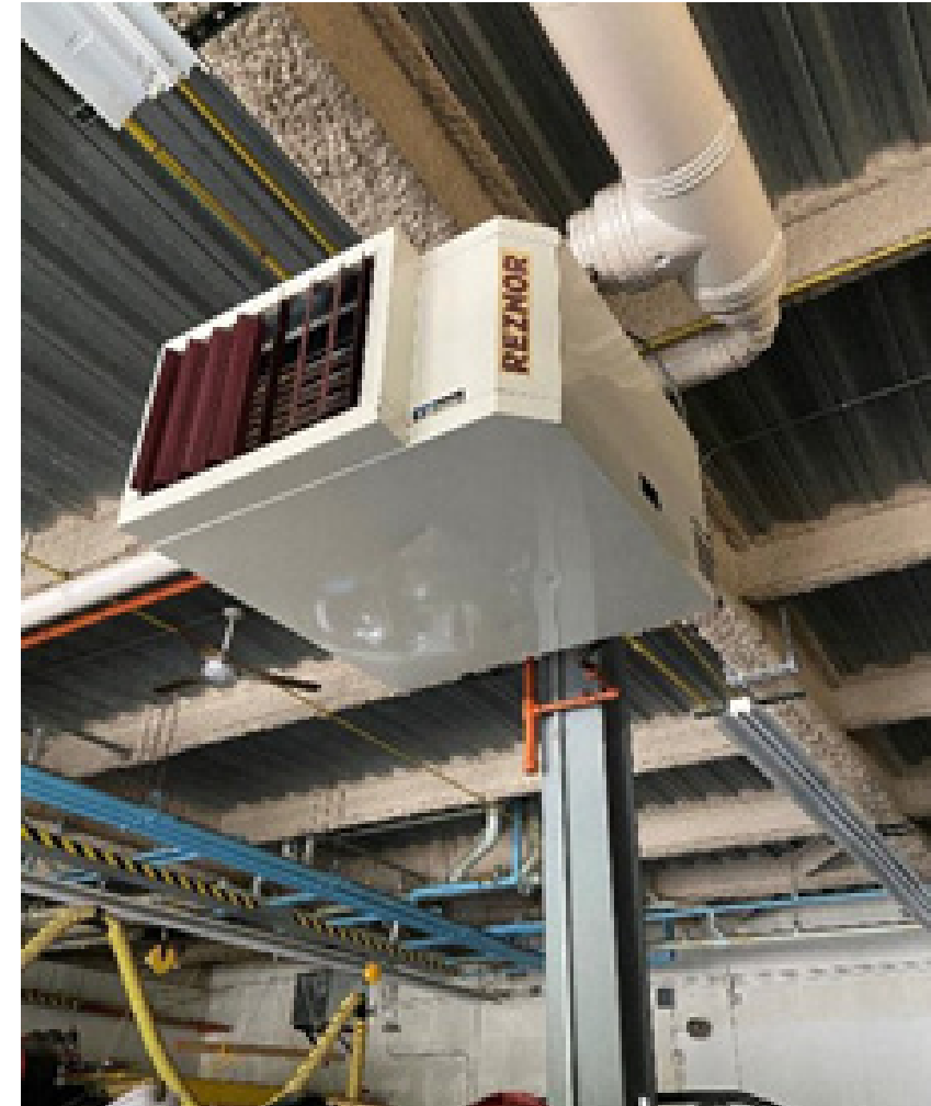
Gas Fired Unit Furnace
