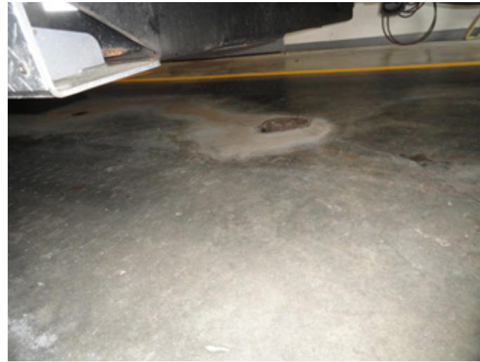
Photo #10 Basement Apparatus Room slab Shrinkage cracks at the front north bay
