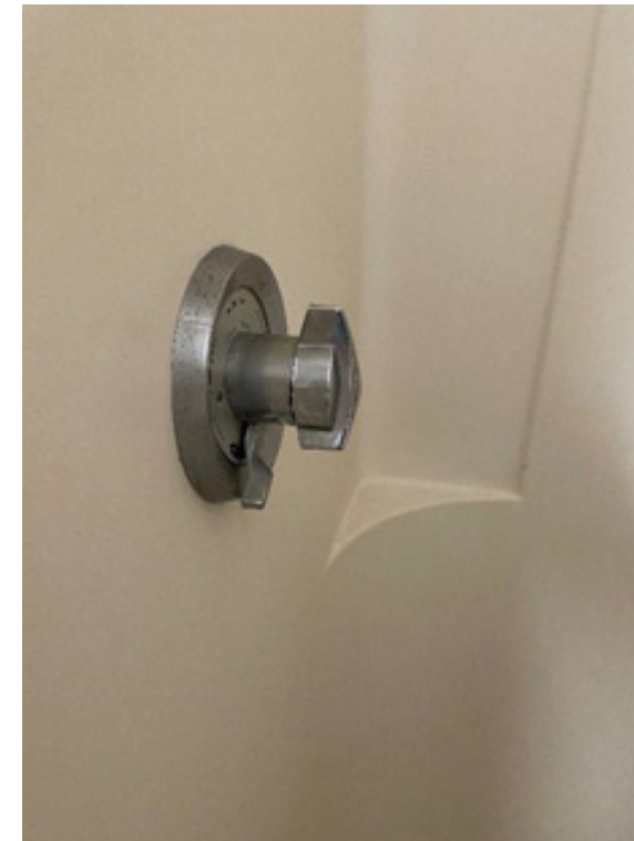
Existing Shower Valve
