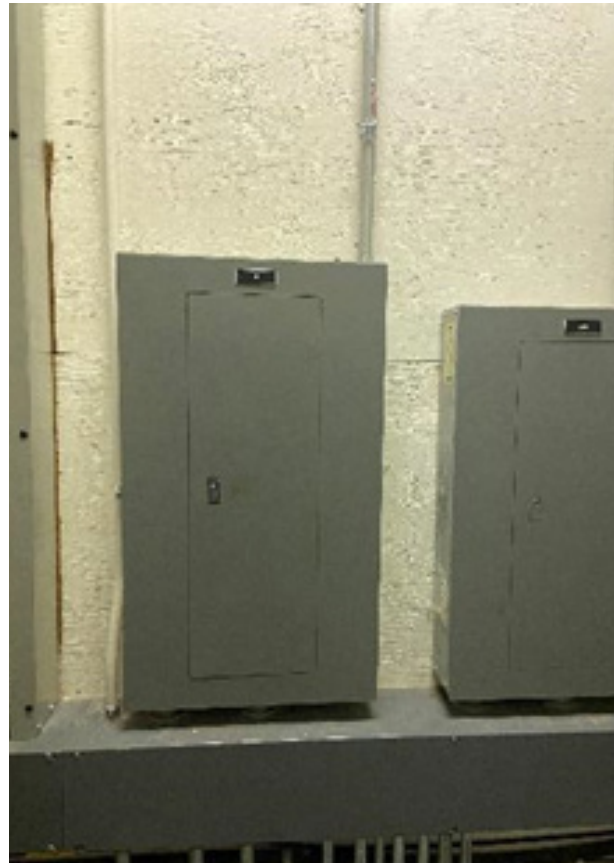
Older Electrical Panels
