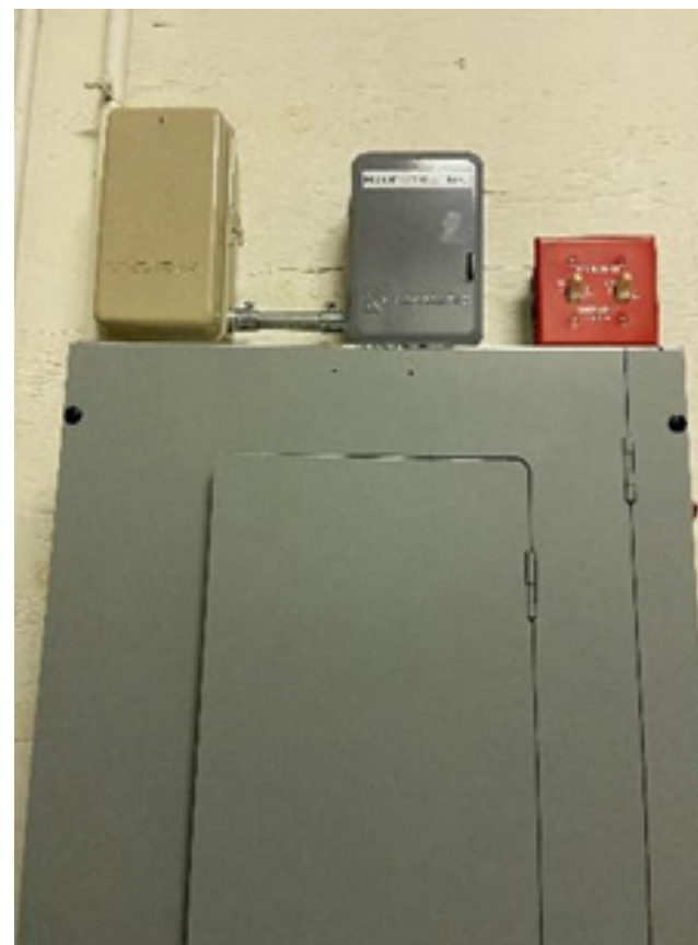
Newer Electrical Panel
