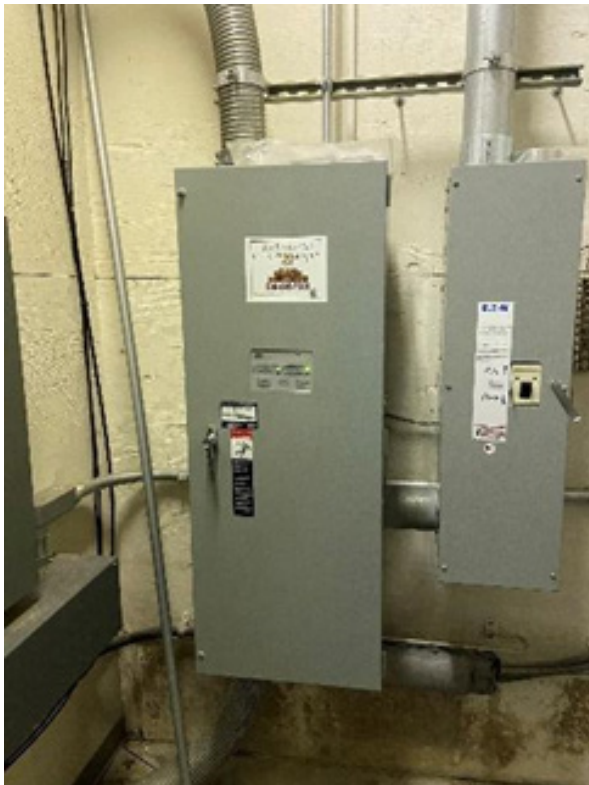
Automatic Transfer Switch
