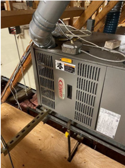
Furnace Unit in Attic Space
