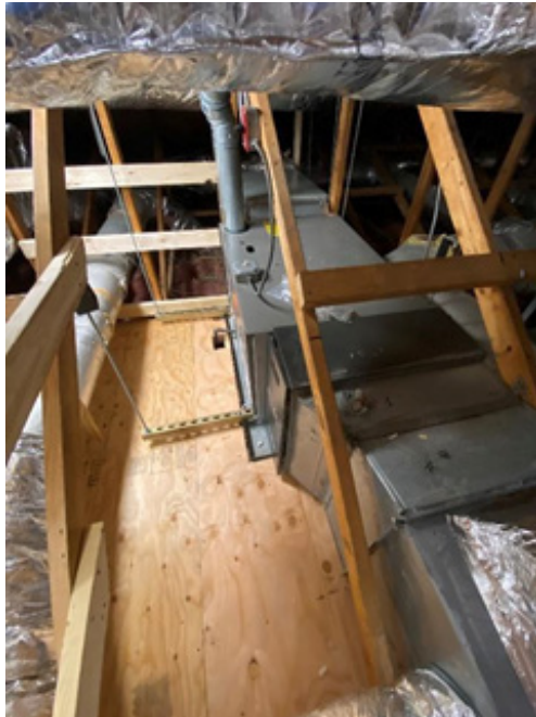
Furnace Unit in Attic Space
