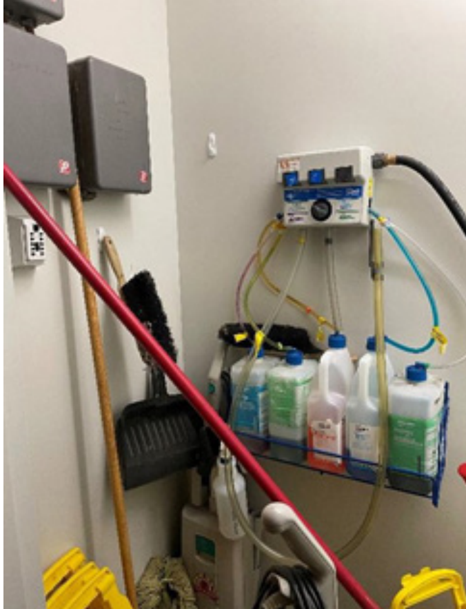
Chemical Dispensing Unit
