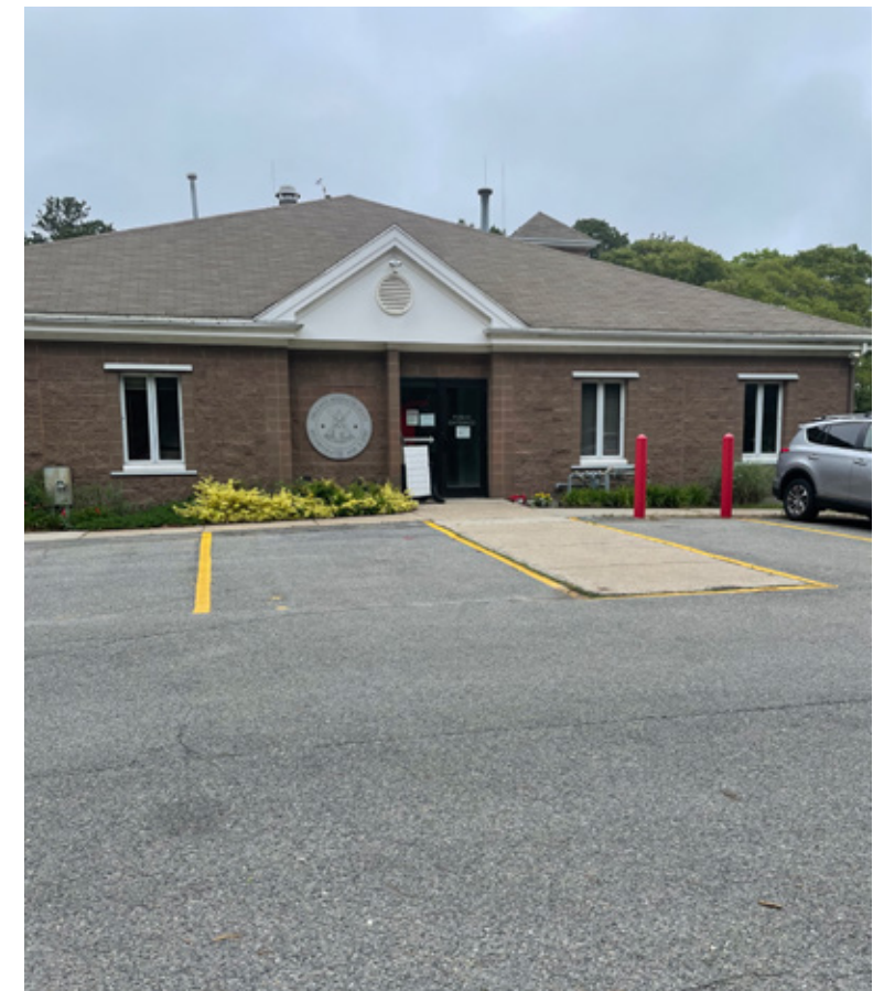
Main Entry to building is not clear, and access has non-compliant slope
