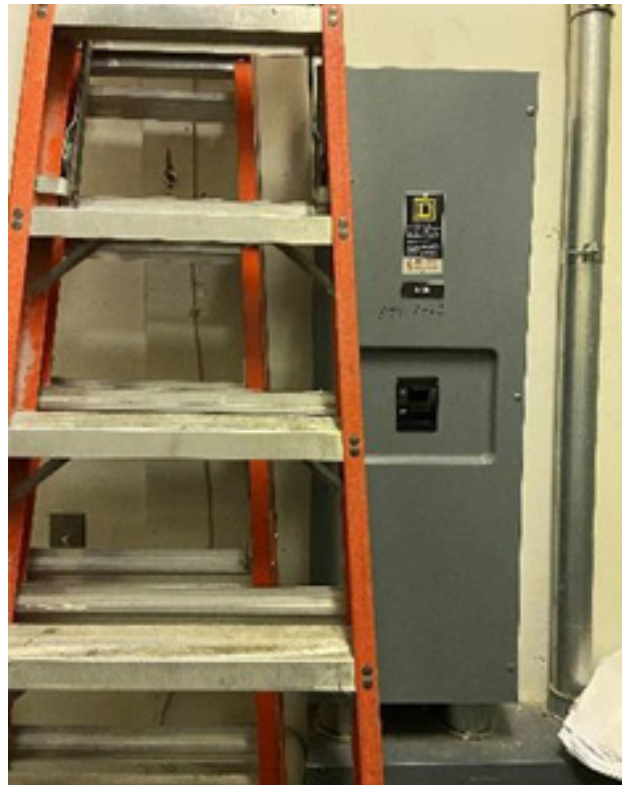
Electrical Service Equipment
