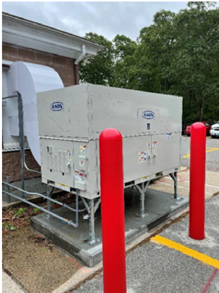
Outdoor Energy Recovery Ventilator (ERV)
