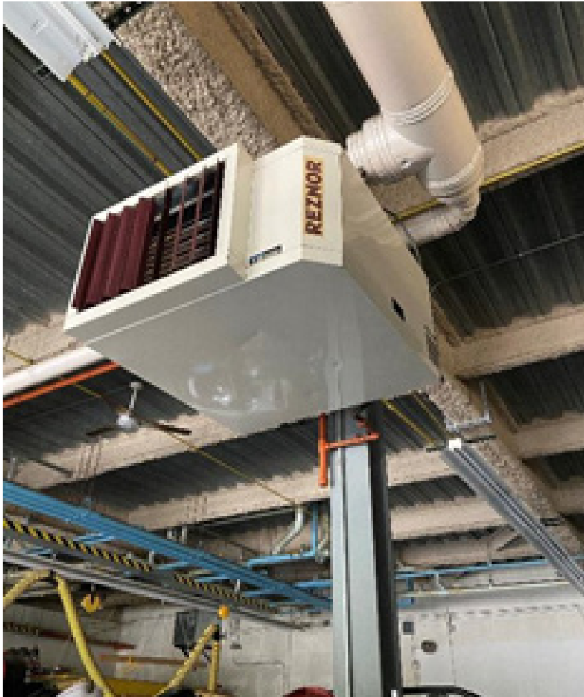
Gas Fired Unit Furnace
