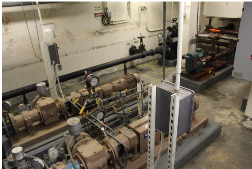
Intermediate Pumps Requiring Rebuild
