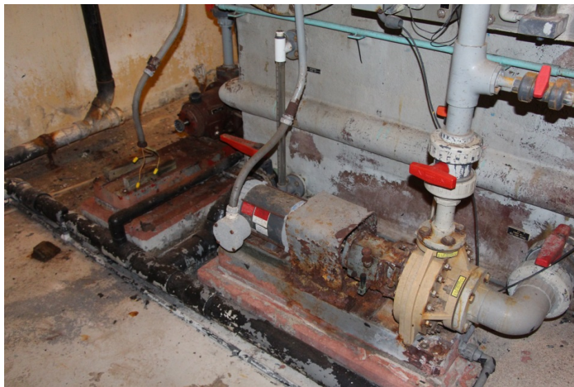
Main Odor Control Wet Scrubber Recirc Pump
