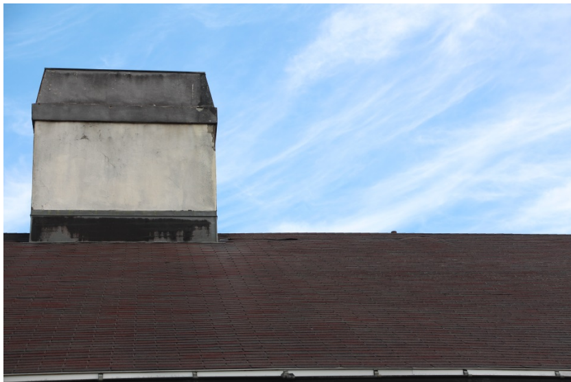
Admin Building Roof (Bulge to right of vent)
