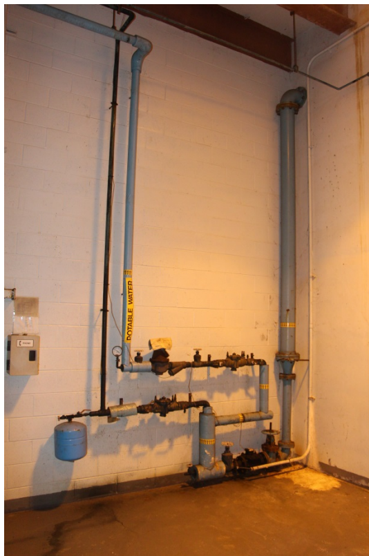
Corrosion in Potable Water Piping
