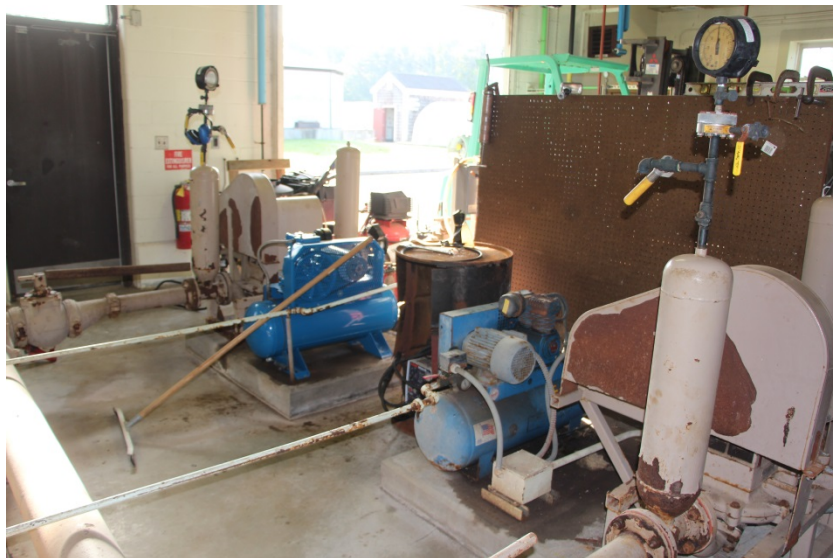
Thickened Sludge Pumps in Need of Component Repair/Replacement
