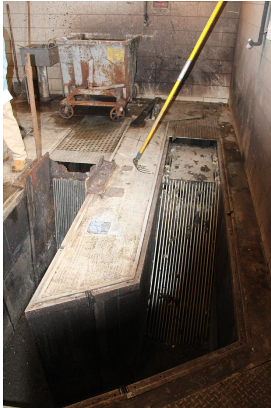
Severe Corrosion on Receiving Area Screen
