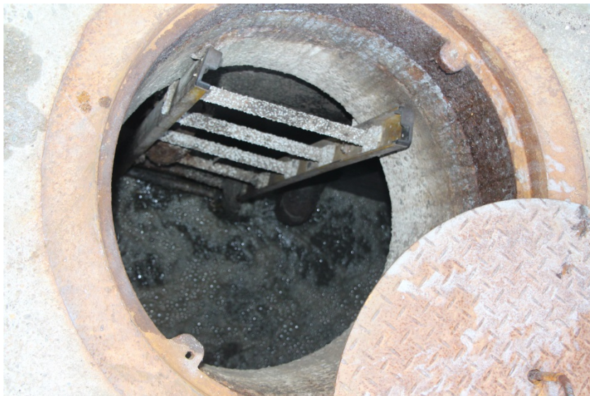
Septage Equalization Tank Diffused Air Mixing
