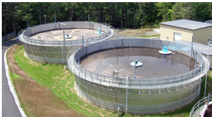
Figure 2: Sequencing Batch Reactors (Aqua-Aerobic Systems, Inc.)
