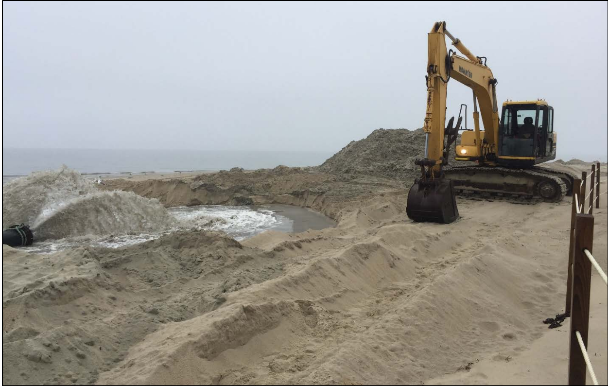
Figure 15. BCD excavator managing dredged materials at the dewatering site on Cold Storage Beach, Dennis, MA during active operations on February 13, 2020.
