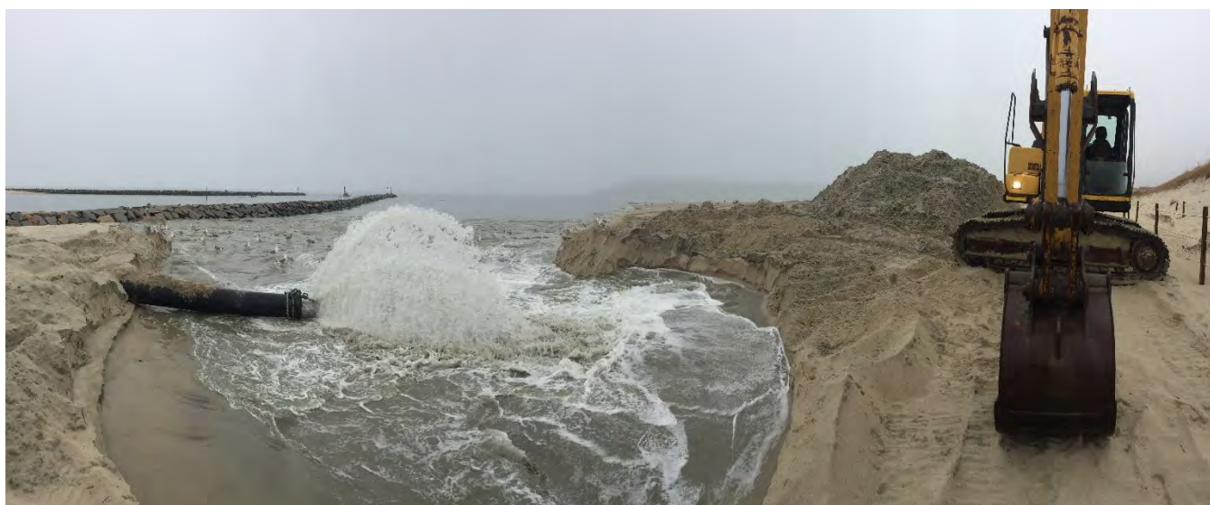
Figure 2 – Active dewatering site on Cold Storage Beach. County dredge visible in background between jetties.
