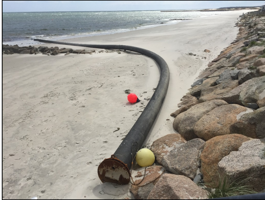
Figure 9. Length of HPDE discharge pipe coming ashore at local dewatering area, Yarmouth, MA, May 2019.
